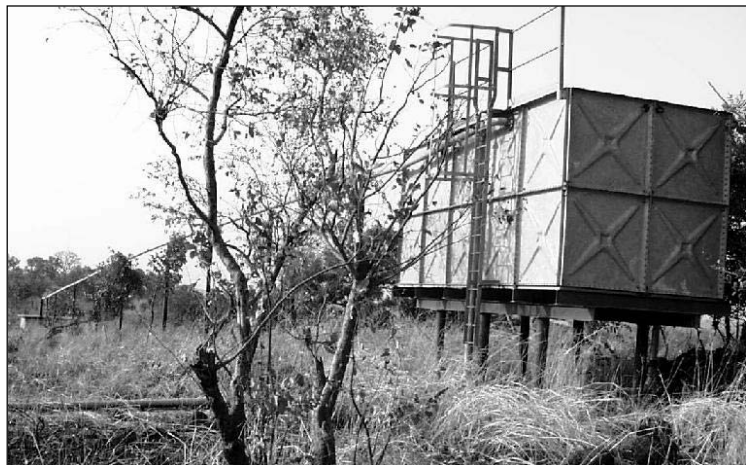
Figure 14: Header tank of the reticulated water supply system which has been the greatest issue regarding sustainability of the relocation process
